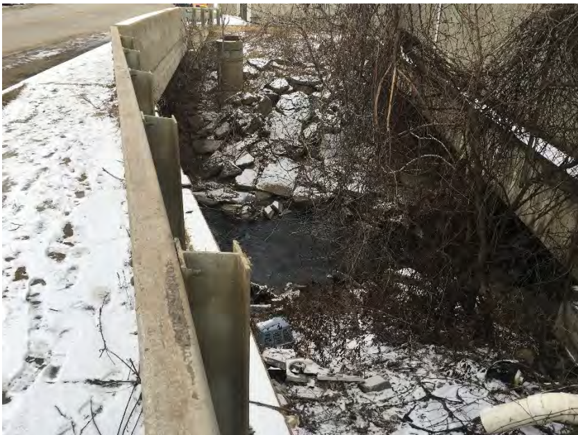
Photo: 4 Date: December 18, 2019 Description: East side of bridge, facing north along the northbound lane of Seminary Street.
