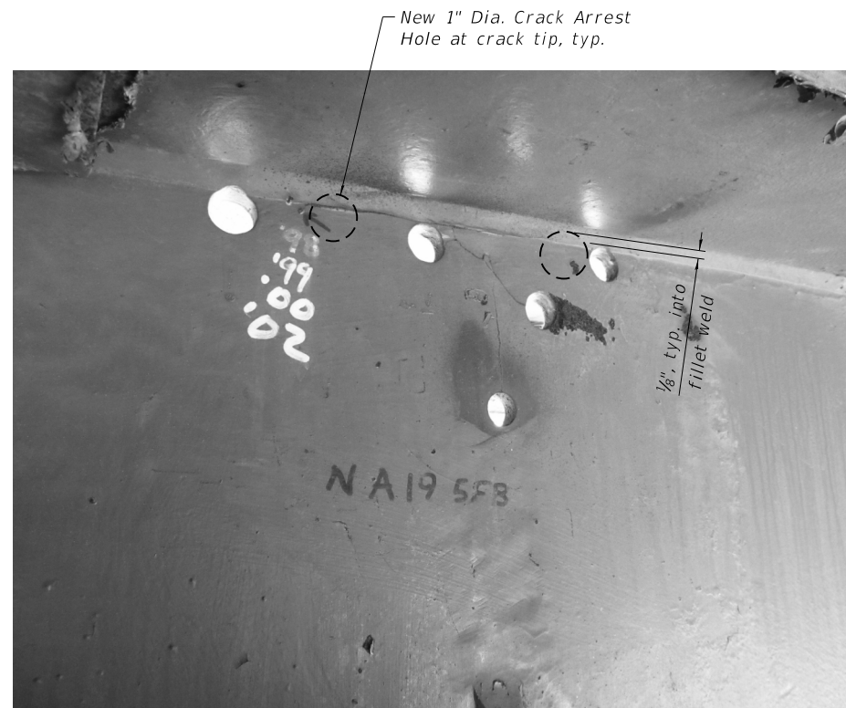
SPAN A19 CRACK ARREST HOLES Girder A1 at first interior floor beam from Pier A20
