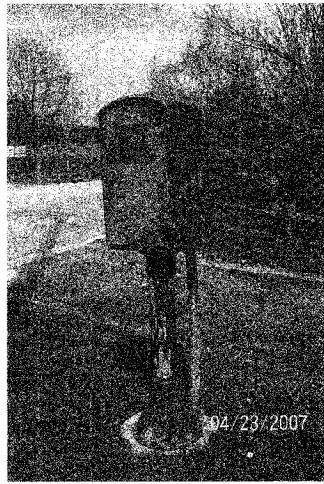
1 EXISTING PEDESTAL MOUNTED CONTROLLER NOT TO SCALE
