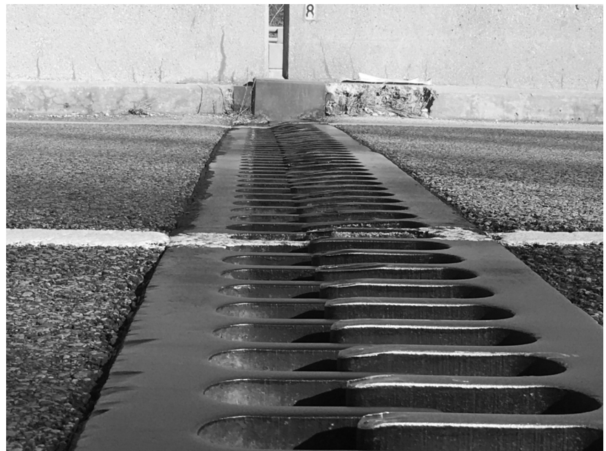
FINGER PLATE AT PIER 8
