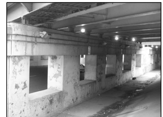
EXISTING LIGHTING: PIER 2 (Looking Northwest)
