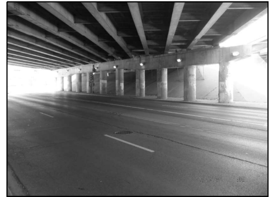
EXISTING LIGHTING PIER 1 (Looking Northwest)
