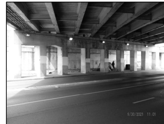
EXISTING LIGHTING: PIER 2 (Looking Northwest)
