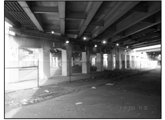
EXISTING LIGHTING: PIER 1 (Looking Northwest)
