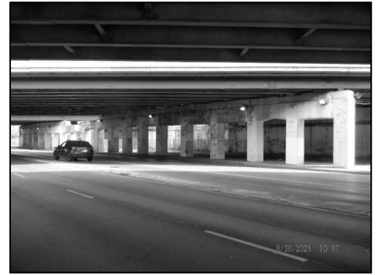
EXISTING LIGHTING: PIER 1 (Looking Northeast)
