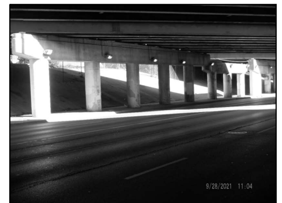
EXISTING LIGHTING PIER 1 (Looking Northeast)
