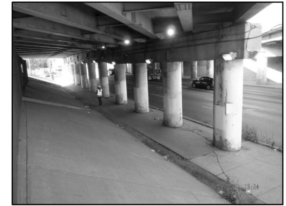
EXISTING LIGHTING PIER 2 (Looking Northwest)
