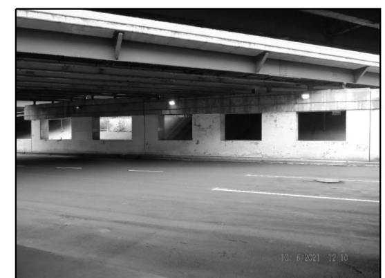
EXISTING LIGHTING: PIER 2 (Looking Northeast)
