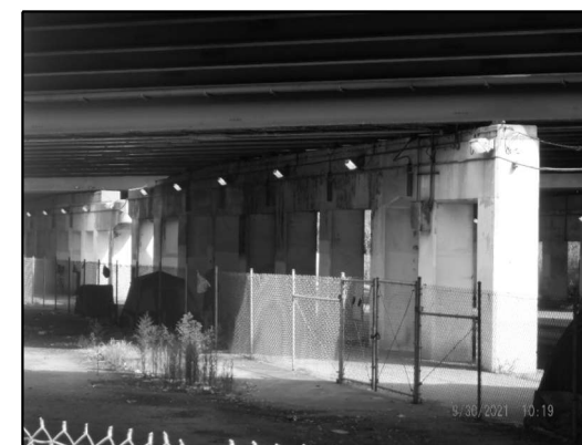
EXISTING LIGHTING: PIER 2 (Looking Northeast)
