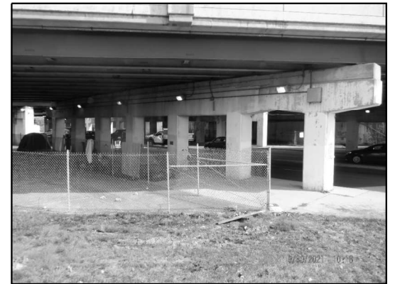
EXISTING LIGHTING: PIER 2 (Looking Northeast)
