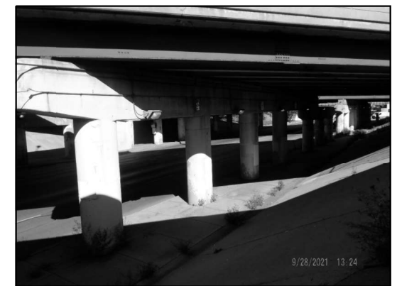
EXISTING LIGHTING PIER 2 (Looking Northeast)
