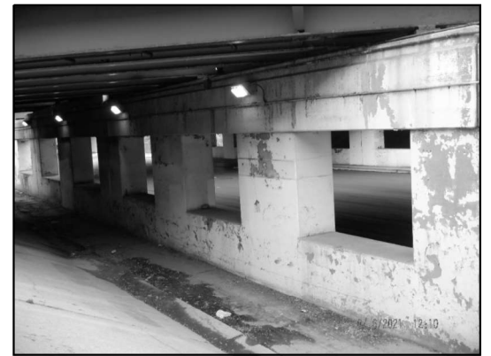
EXISTING LIGHTING: PIER 1 (Looking Northeast)
