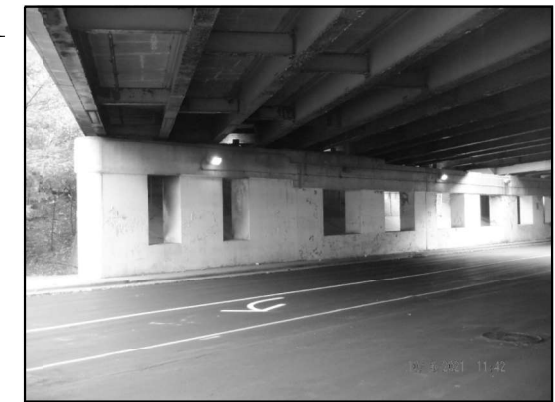
EXISTING LIGHTING: PIER 1 (Looking Northwest)
