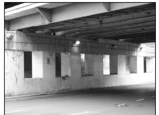
EXISTING LIGHTING: PIER 1 (Looking Northwest)
