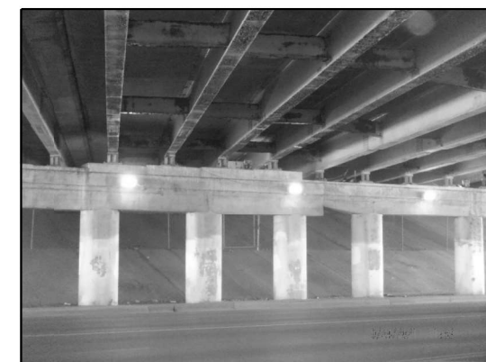
EXISTING LIGHTING: PIER 2 (Looking Southeast)
