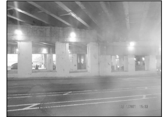
EXISTING LIGHTING: PIER 3 (Looking Southwest)
