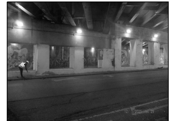
EXISTING LIGHTING: PIER 3 (Looking Southeast)
