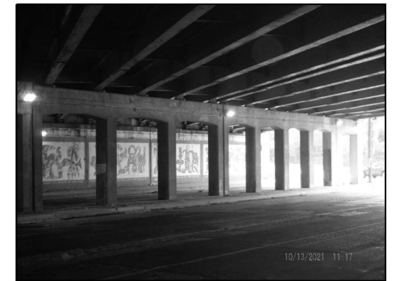
EXISTING LIGHTING: PIER 1 (Looking Southeast)
