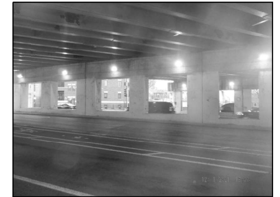
EXISTING LIGHTING: PIER 3 (Looking Southwest)
