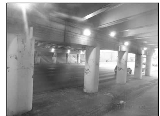
EXISTING LIGHTING: PIER 1 (Looking Southeast)
