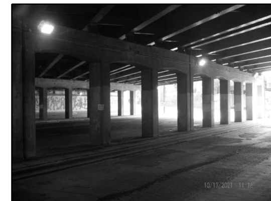
EXISTING LIGHTING: PIER 2 (Looking Southeast)
