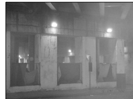
EXISTING LIGHTING: PIER 2 (Looking Northwest)
