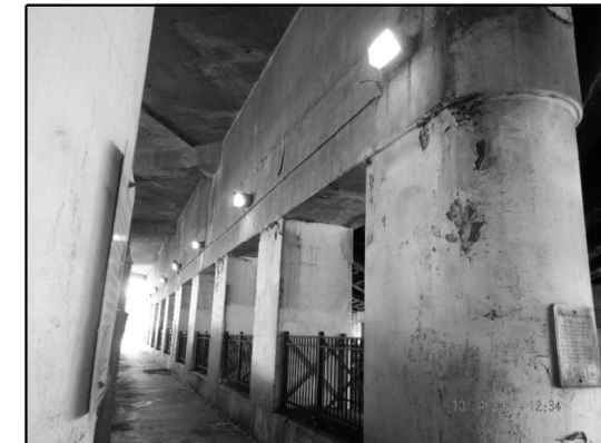
EXISTING LIGHTING: PIER 1 (Looking Northwest)
