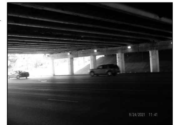
EXISTING LIGHTING: PIER 1 (Looking Southwest)
