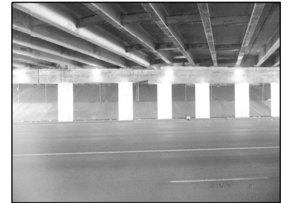
EXISTING LIGHTING: PIER 1 (Looking Northwest)
