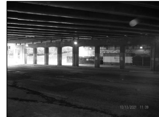
EXISTING LIGHTING: PIER 2 (Looking Southwest)
