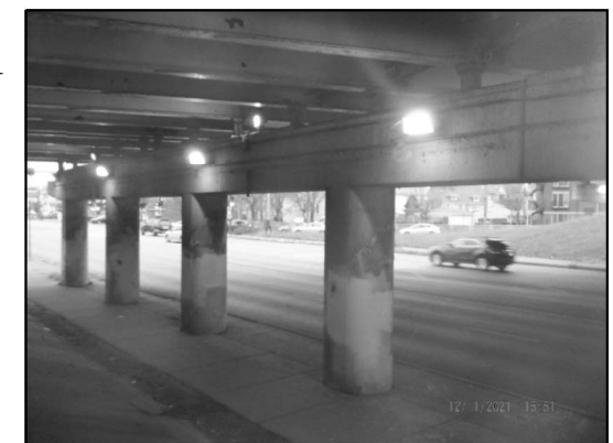
EXISTING LIGHTING: PIER 2 (Looking Southwest)
