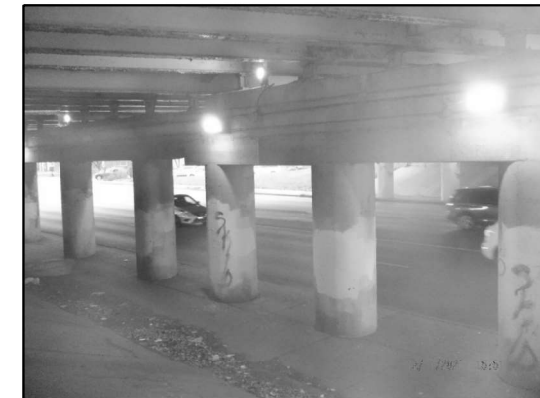
EXISTING LIGHTING: PIER 2 (Looking Southwest)
