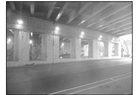
EXISTING LIGHTING: PIER 3 (Looking Southeast)
