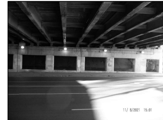
EXISTING LIGHTING: PIER 1 (Looking Southwest)
