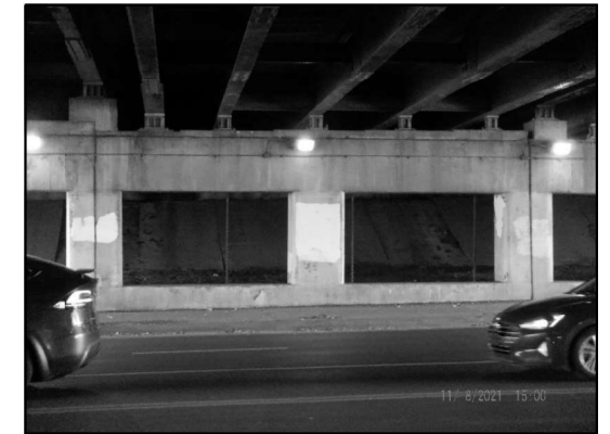
EXISTING LIGHTING: PIER 1 (Looking Southwest)
