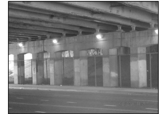
EXISTING LIGHTING: PIER 1 (Looking Southeast)
