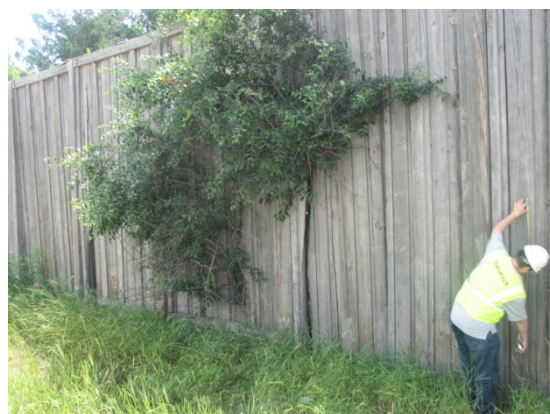
Photo 6. Four Sequential Damaged Panels (NAW 2)
