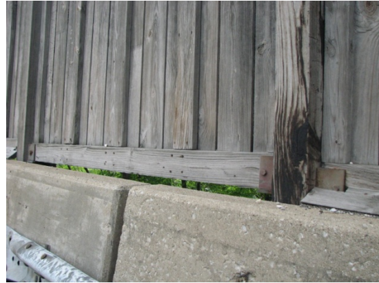
Photo 2. Missing Bottom Gap Board at SN 016-1134 (NAW 1)
