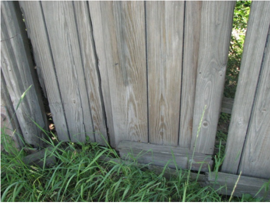
Photo 7. Failed Connection and Severed Foundation Plank (NAW 2)
