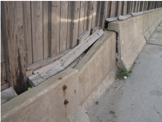
Photo 3. Settled Parapet & Damaged Bot. Gap Board & Fdn. Plank (NAW 1)
