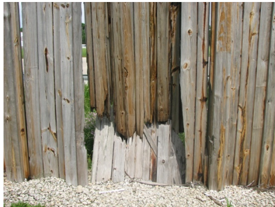
Photo 17. View of Damaged Panel from Residential Side (NAW 5)
