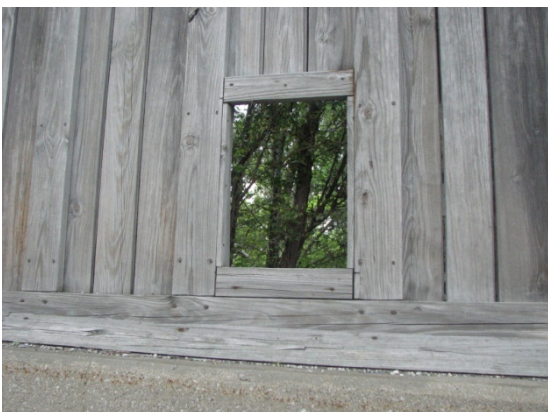
Photo 11. Missing Access Hole Door (NAW 2)
