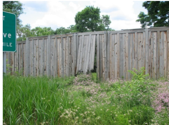
Photo 16. View of Damaged Panel (NAW 5)
