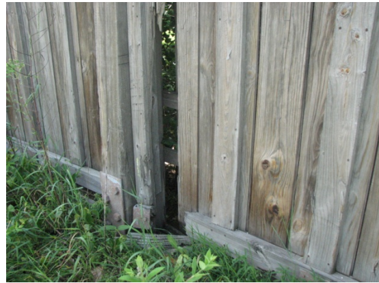
Photo 10. Failed Joint Connection (NAW 2)
