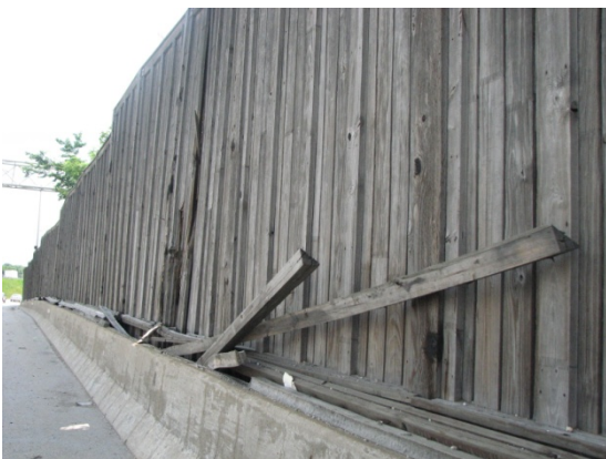
Photo 5. Damaged Bottom Gap Boards on top of Geofoam (NAW 1)
