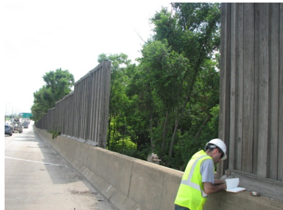
Photo 12. Three Missing Panels at SN 016-1133 (NAW 2)
