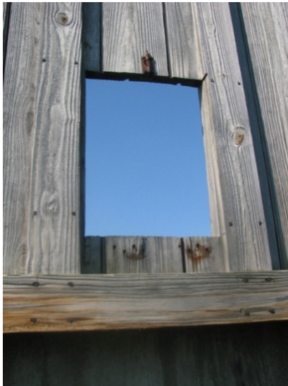
Photo 15. Missing Access Hole Door (NAW 4)
