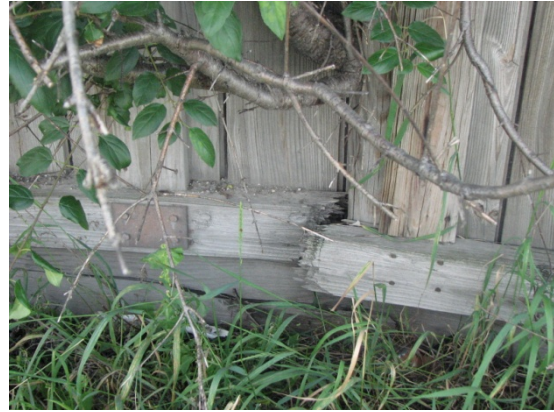
Photo 8. Severed Foundation Plank (NAW 2)
