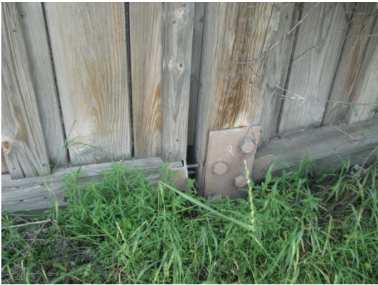
Photo 9. Failed Joint Connection (NAW 2)
