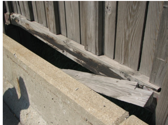
Photo 4. Damaged Fdn. Plank (NAW 1)
