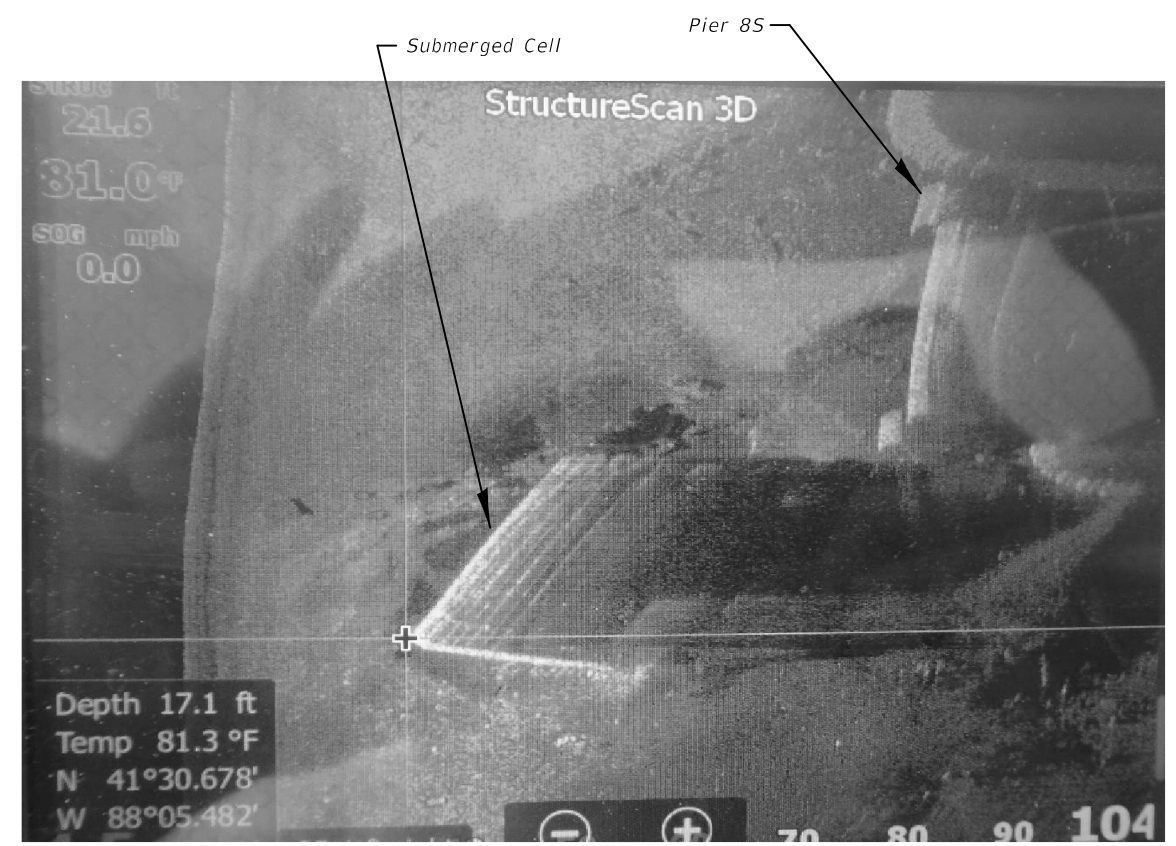
SIDE SCAN PHOTO SHOWING EXISTING SUBMERGED CELL (For existing details, see sheet 6A of 6)
