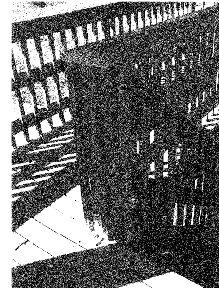
Photo 17 - Loose Railing End Posts (Typical)
