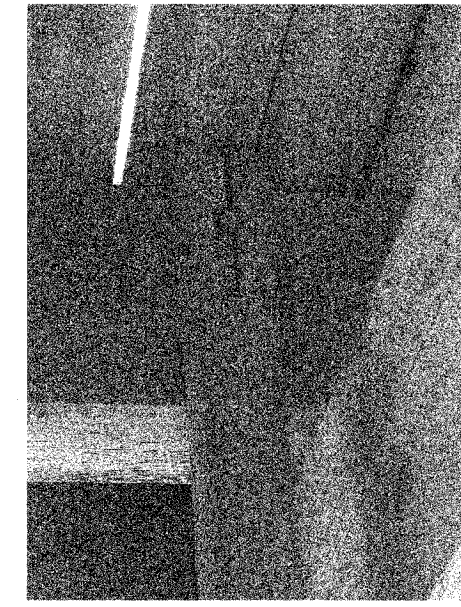
Photo 18 - Split Hanger at Top Support (Typical)
