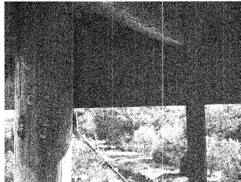
Photo 09- (Second Level) 8"x16" Beam at East Side showing Horizontal cracks at Mid Depth for the Full Length
