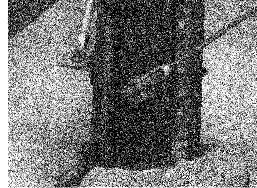
Photo 05- Wood Treatment leaching out of the Tower Structure and accumulating at Pole Base.
