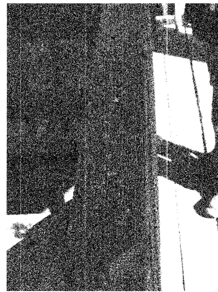
Photo 16 - Railing Showing very Rough surface and Loose Splinters
