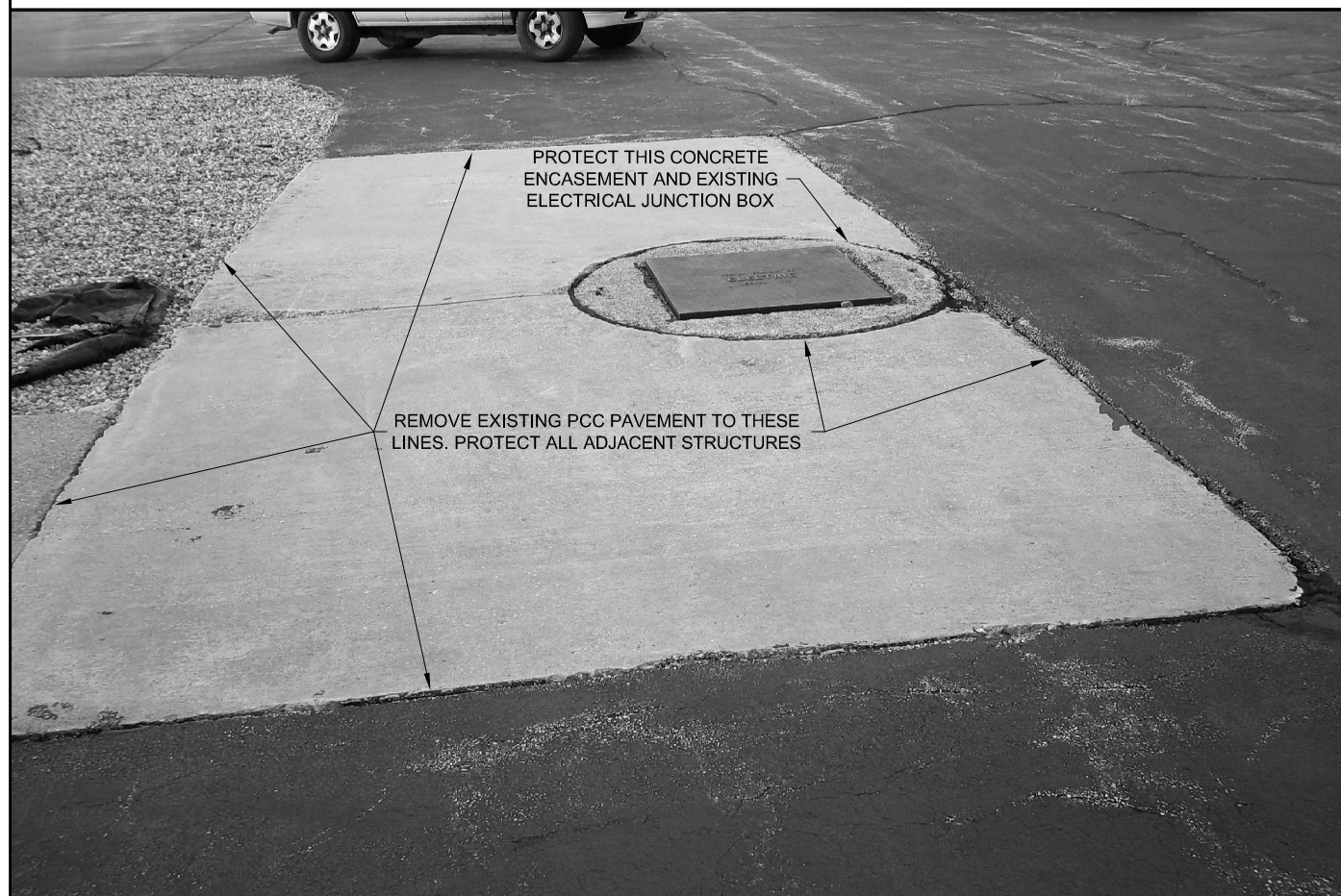
GOLF RAMP - EXISTING ELECTRICAL JUNCTION BOX
