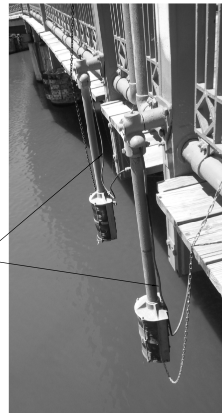
CENTER SPAN NAVIGATION LIGHTS
