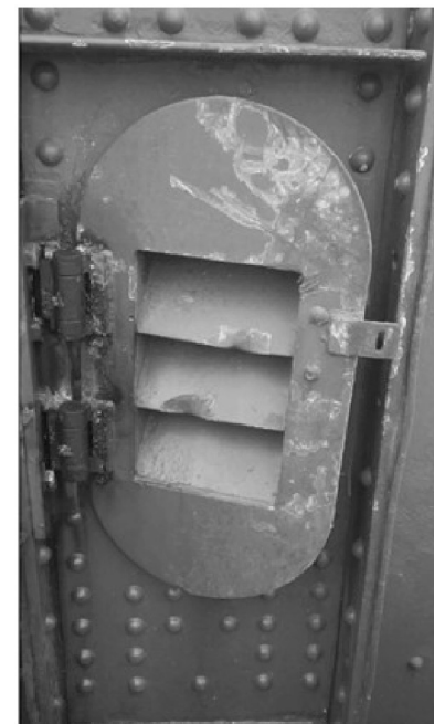
EXISTING ACCESS DOOR PHOTO
