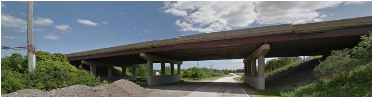
Photo 2: View of IL Rte 120 Bridge over Old Skokie Road and the UPRR railroad, facing south.
