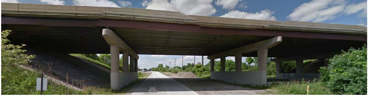
Photo 1: View of IL Rte 120 Bridge over Old Skokie Road and the UPRR railroad, facing north.
