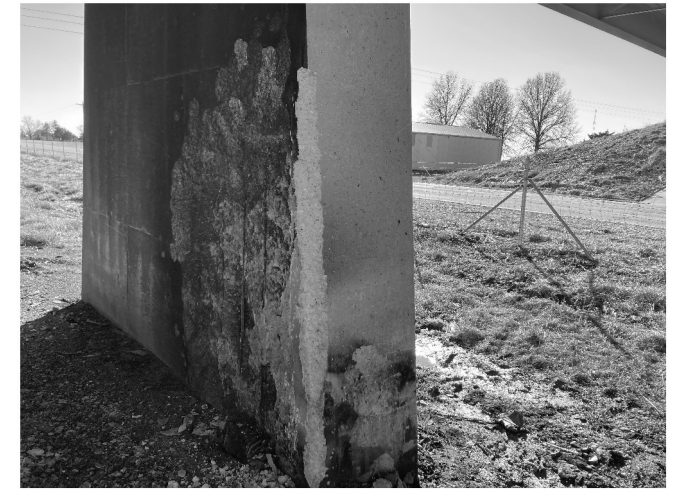
EXISTING PIER DAMAGE TO BE REPAIRED
