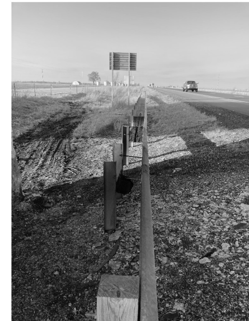
DAMAGED GUARDRAIL BLOCKS TO BE REPLACED
