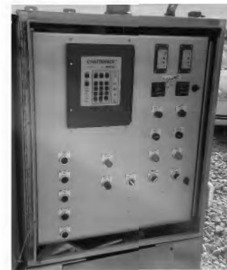
I-70 REST AREA W/B PUMP STATION EXISTING DIALER PHOTO
