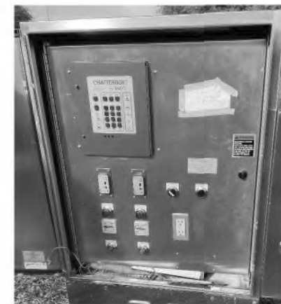
I-64 REST AREA W/B PUMP STATION EXISTING DIALER PHOTO
