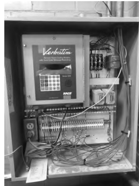
25TH STREET PUMP STATION EXISTING DIALER PHOTO
