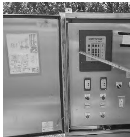
I-64 REST AREA E/B PUMP STATION EXISTING DIALER PHOTO
