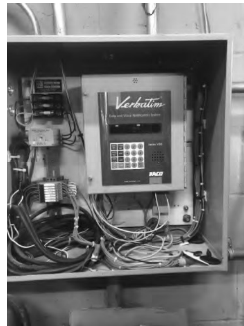
VENICE PUMP STATION EXISTING DIALER PHOTO
