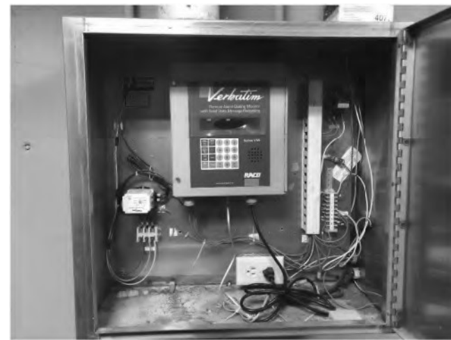
MCCAMBRIDGE PUMP STATION EXISTING DIALER PHOTO
