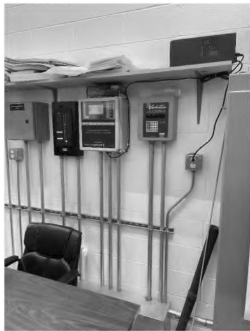
MISSOURI AVENUE PUMP STATION EXISTING DIALER PHOTO
