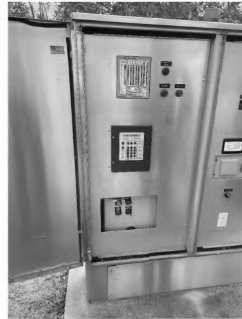
I-55 REST AREA N/B PUMP STATION EXISTING DIALER PHOTO
