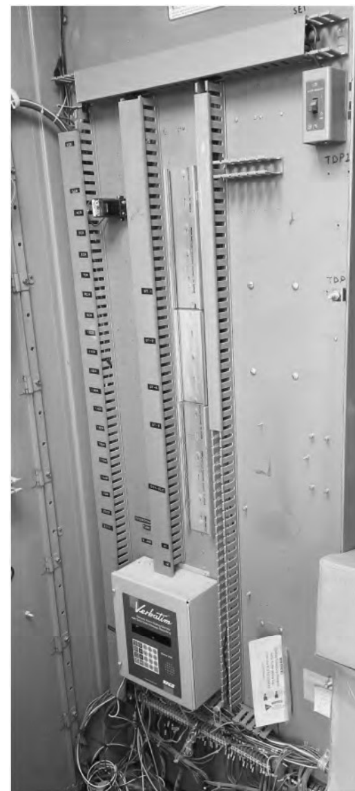
COLLINSVILLE #1 PUMP STATION EXISTING DIALER PHOTO
