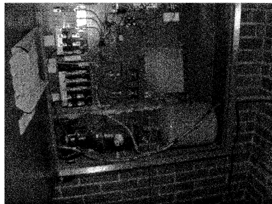
4 BOILER TO BE DEMOLISHED ON LEVEL THREE (WEST) Scale: None Cost included in the cost of HVAC Demolition (Mechanical and Electrical).
