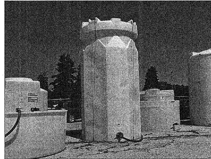
LARGE DEICING STORAGE TANKS
