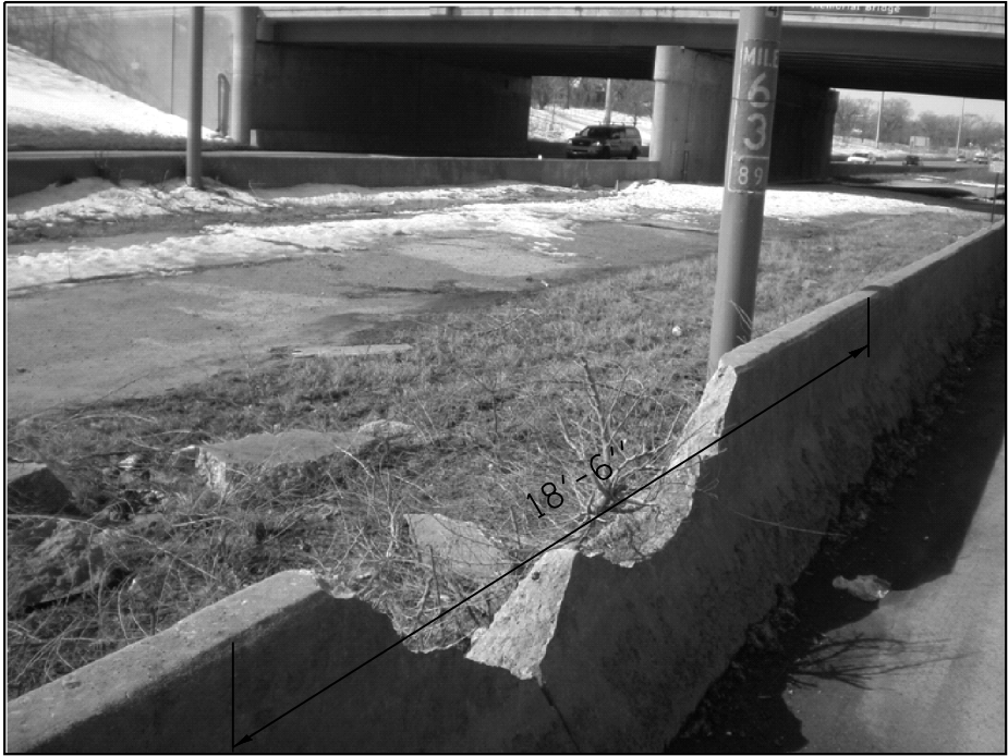
HALF DEPTH REPAIR REPLACE 18 1/2' OF BARRIER WALL FOR MORE DETAILS, SEE SHEET #6
