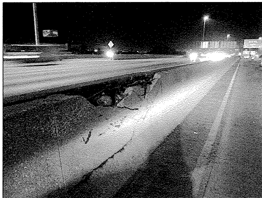
CENTER PARAPET REPAIR LOOKING SOUTH FACING SOUTHBOUND PARAPET FACE FOR MORE DETAILS, SEE SHEET #7
