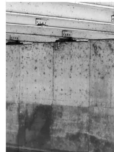
SPALL AT SOUTH FACE
