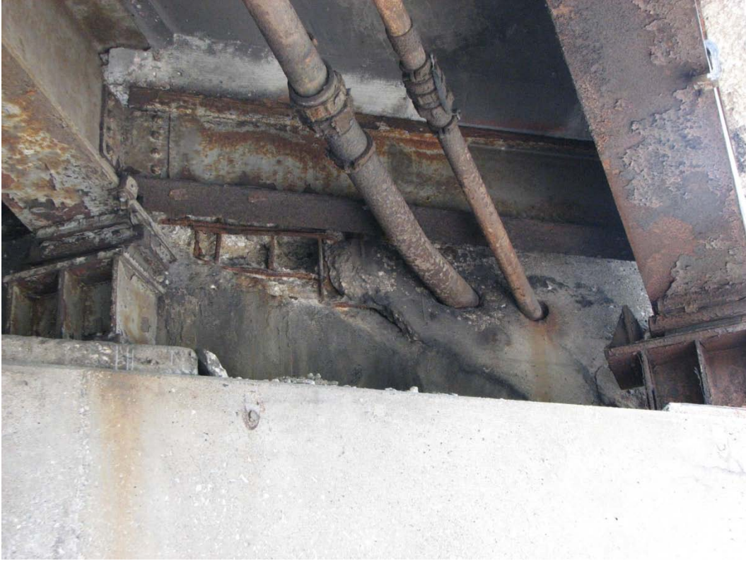
Photo 7 – Abutment Backwall Spalling and Utilities
