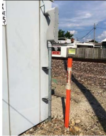
Exterior hut fiber entrance
