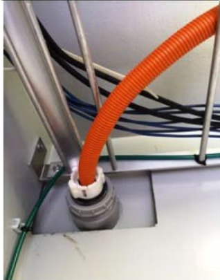
Interior hut fiber entrance
