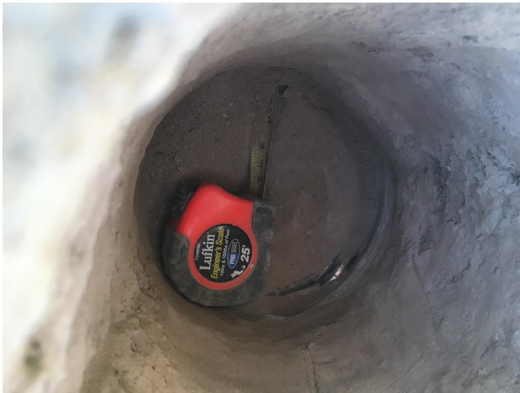
Photo 4) Steel obstruction encountered in attempt #6. (November 20, 2017)
