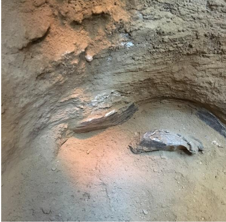
Photo 3) Steel obstruction encountered in attempt #5. (November 20, 2017)
