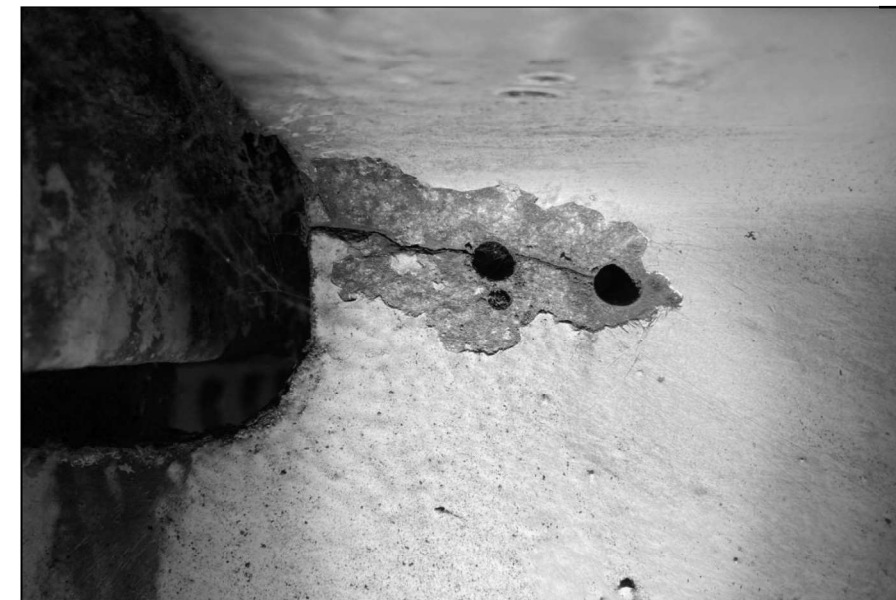
Stringer 1 at Floor Beam FB0' upper web crack that was arrested, no further propagation
