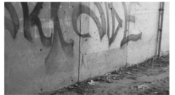
CRACKS ON PIER 2 (NF) (Looking South)
