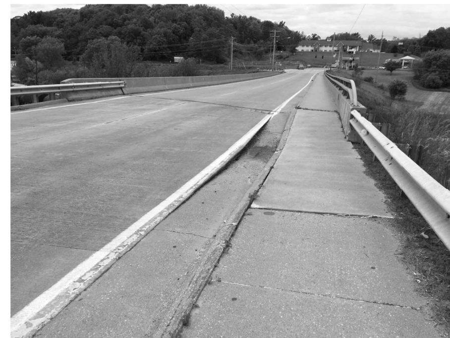
SOUTH EAST APPROACH DAMAGE
