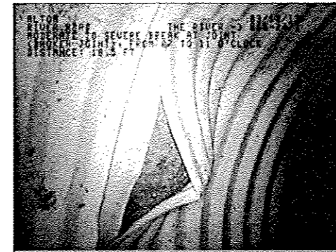
PHOTO FROM 03/13/2012 VIDEO OF PIPE SHOWING DAMAGED JOINT LOCATED APPROXIMATELY 18.5 FEET UPSTREAM FROM THE OUTLET. REPAIR SHALL BE PERFORMED FROM INSIDE THE PIPE. OPEN EXCAVATION WILL NOT BE ALLOWED.
