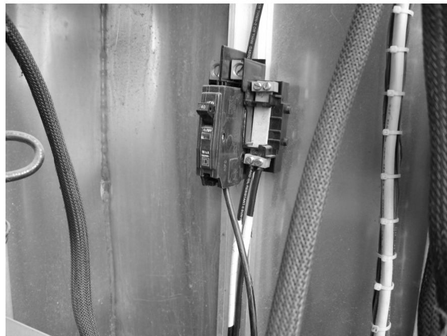
TYPICAL BREAKER INSTALLATION IN SIGNAL/CONTROLLER CABINET
