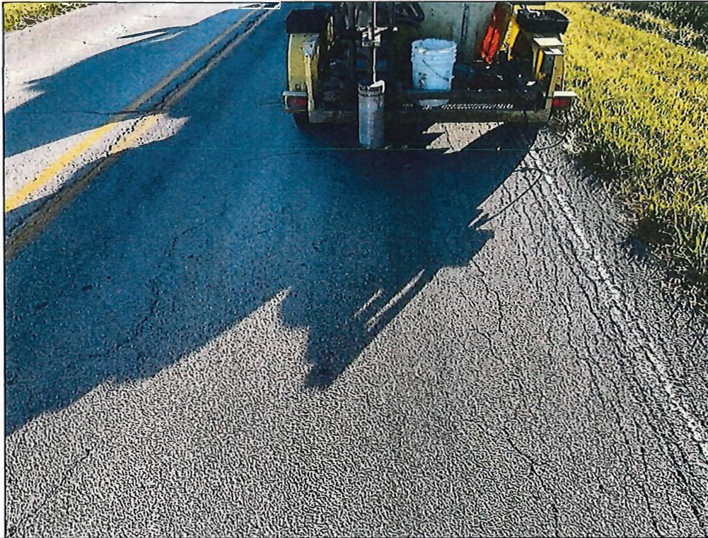
Existing Roadway Condition
