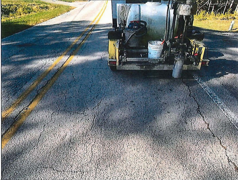
Existing Roadway Condition
