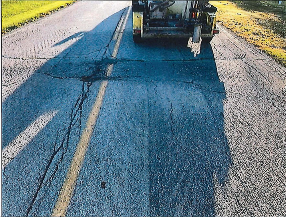
Existing Roadway Condition
