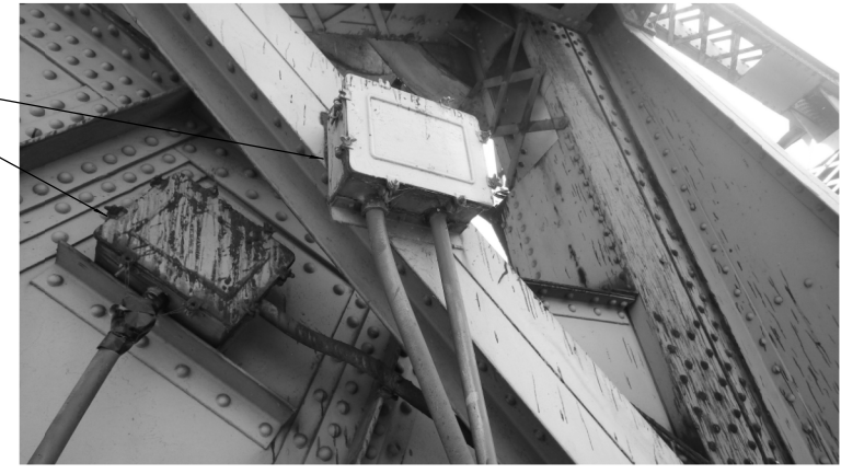
FIXED / MOVABLE SPAN TERMINAL CABINETS (Typical of Jackson Street, Cass Street, Jefferson Street, and McDonough Street Bridges)
