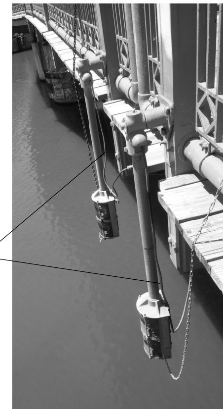
CENTER SPAN NAVIGATION LIGHTS
