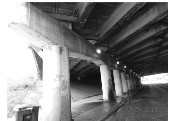
EXISTING LIGHTING: PIER 2 (Looking Southeast)
