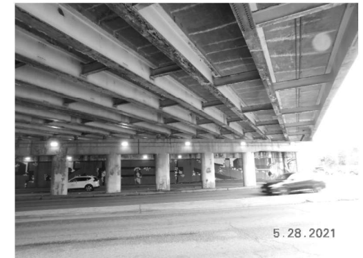
EXISTING LIGHTING: PIER 1 (Looking West)
