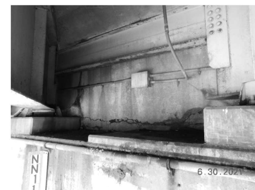
EXISTING ELECTRICAL BOX - SOUTH ABUTMENT (Looking South)
