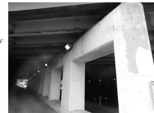
EXIST. LIGHTING: PIER 1 (Looking Southwest)
