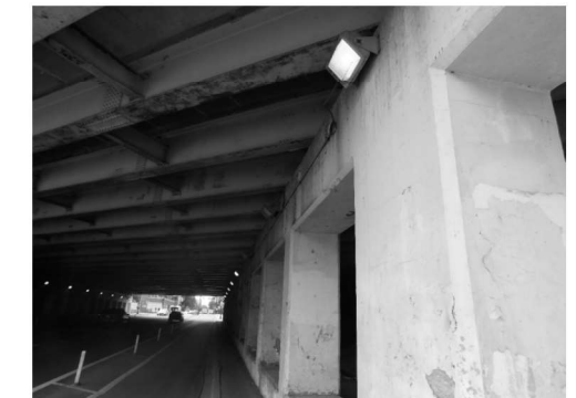
EXIST. LIGHTING: PIER 2 (Looking Southwest)
