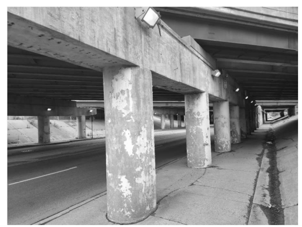
EXISTING LIGHTING: PIER 1 North Face, Looking South
