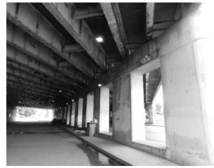
EXISTING LIGHTING - PIER 2 (Looking Northwest)
