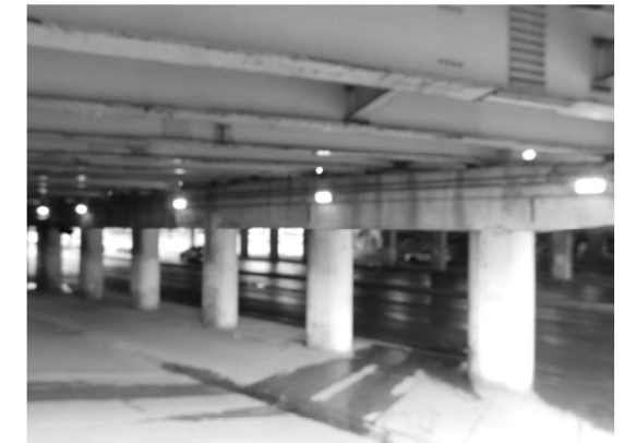
EXISTING LIGHTING: PIER 2 (Looking West)
