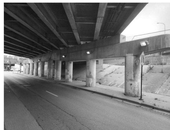
EXISTING LIGHTING: PIER 2 North Face, Looking South
