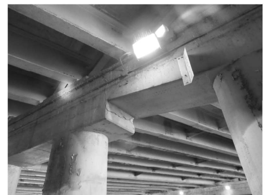
EXISTING LIGHTING: PIER 2 (Looking West)
