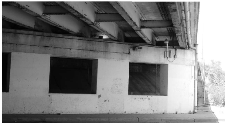
EXISTING LIGHTING: PIER 1 (Looking West)
