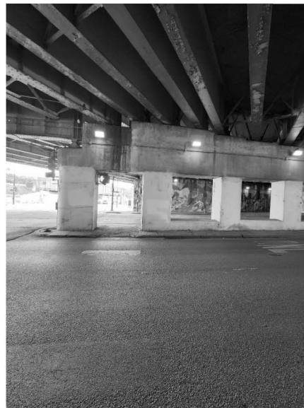
EXISTING LIGHTING: PIER 3 (Looking East)
