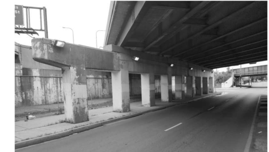
EXISTING LIGHTING: PIER 2 (Looking West)
