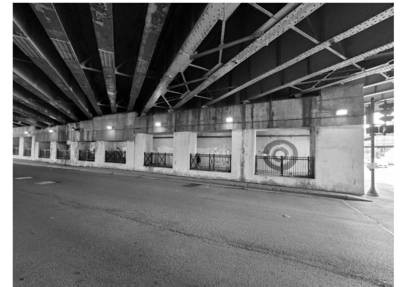
EXISTING LIGHTING: WEST ABUTMENT PIER
