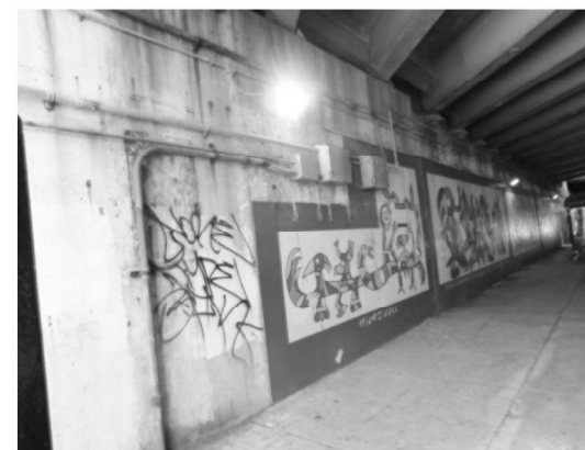
EXISTING LIGHTING: E. ABUT.
