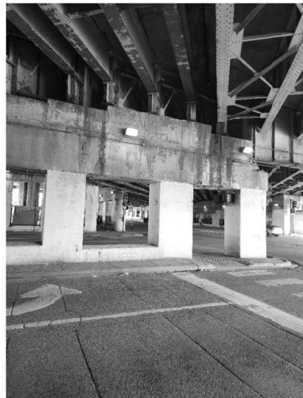
EXISTING LIGHTING: PIER 3 (Looking West)
