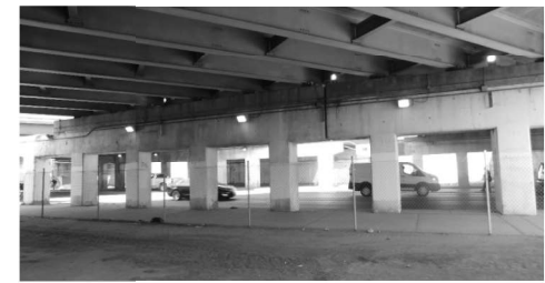
EXISTING LIGHTING: PIER 1 (Looking West)
