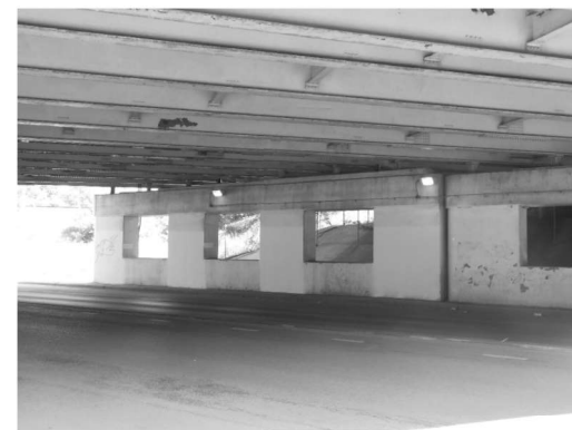
EXISTING LIGHTING: PIER 2 (Looking East)
