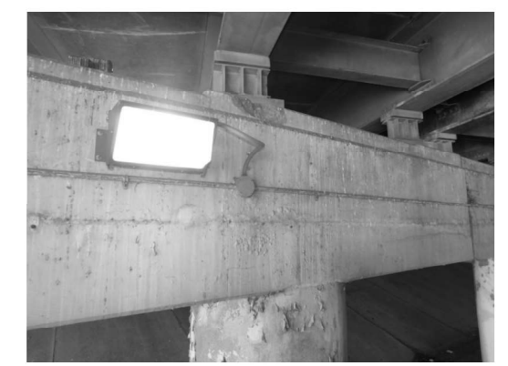
EXISTING LIGHTING: PIER 2 (Looking East)
