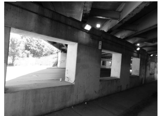
EXISTING LIGHTING: PIER 1 (Looking East)
