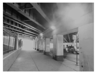
EXISTING LIGHTING: PIER 1 (Looking Southeast)
