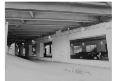
EXISTING LIGHTING: PIER 2 (Looking Southwest)
