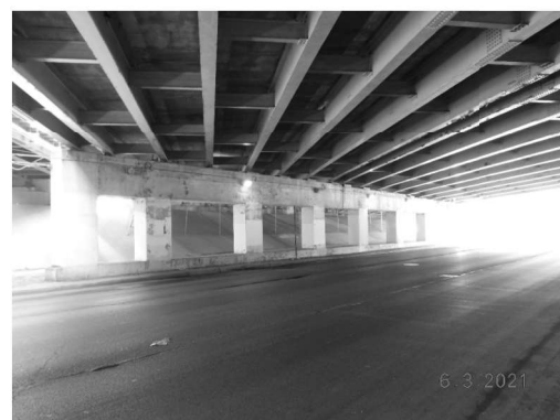
EXISTING LIGHTING: PIER 2 (Looking West)
