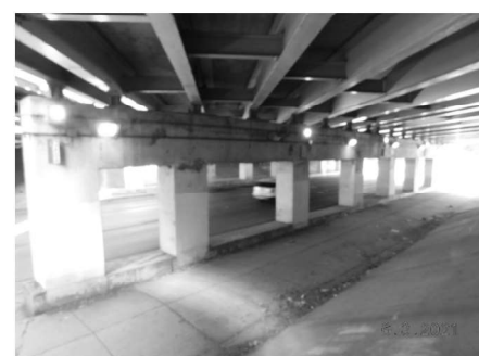
EXISTING LIGHTING: PIER 1 (Looking West)
