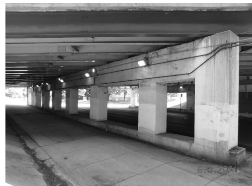
EXISTING LIGHTING: PIER 2 (Looking East)
