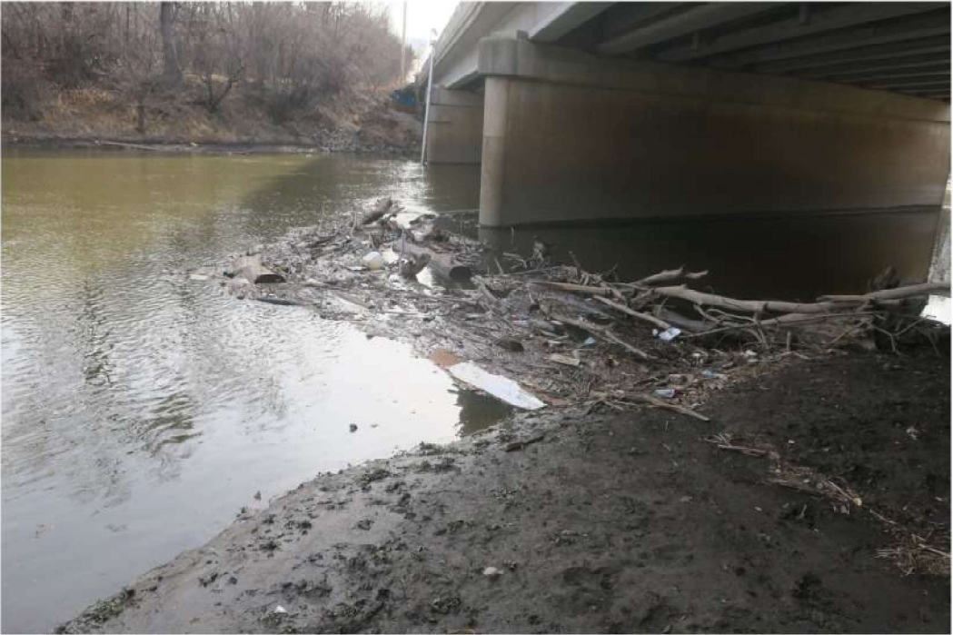
PHOTO 1 - DEBRIS AT PIER 1
