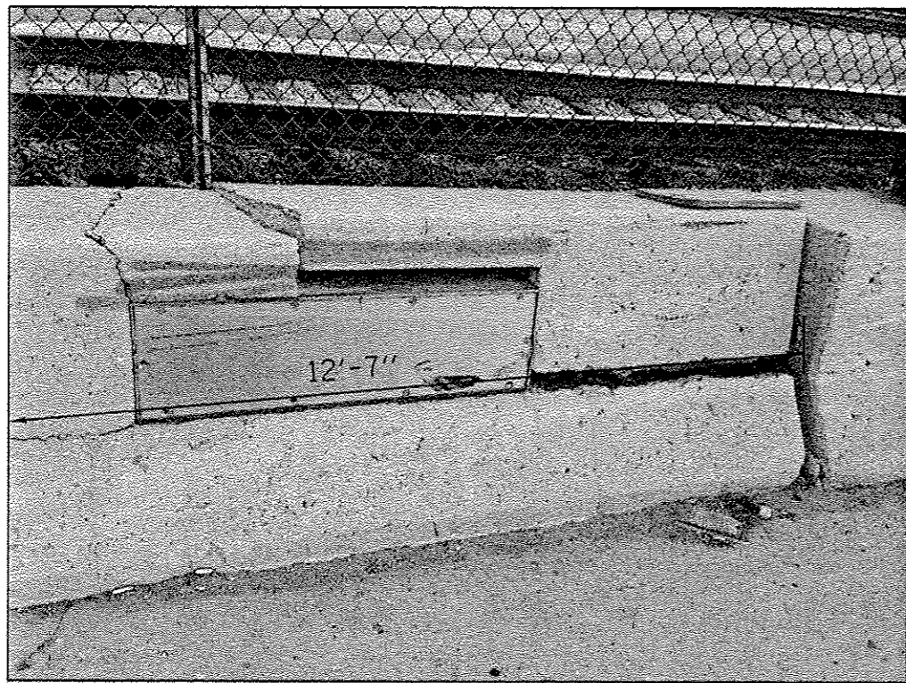
FULL DEPTH REPAIR REPLACE 12'-7" OF BARRIER WALL FOR MORE DETAILS, SEE SHEET #5
