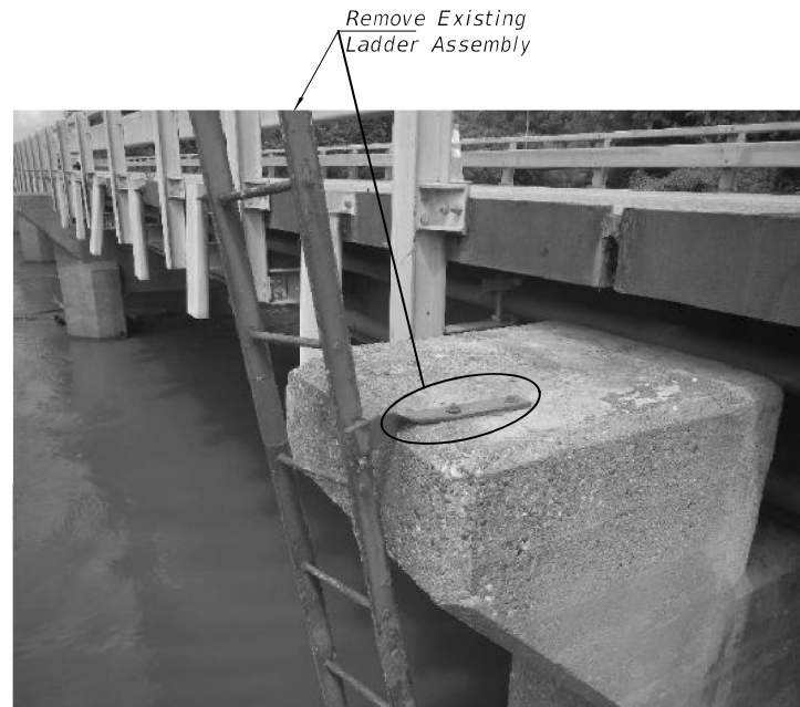
ITEM 512 LADDER REMOVAL Ladder at S. end of Pier 32 (2019 NBIS Photo #532)
