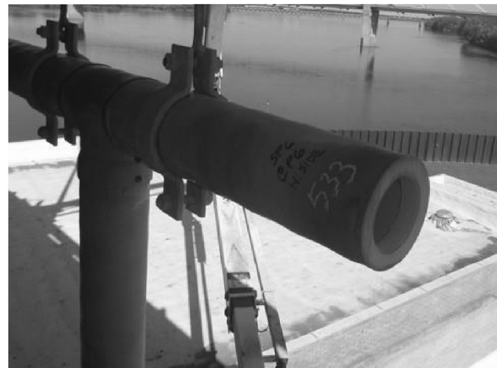
ITEMS 434 & 533 DRAIN CAP REPLACEMENT Item 533 - N. End of Pier 6 (Shown) Item 434 - N. End of Pier 7 (Similar) Cost of New Drain Cap included with Floor Drains. (2015 NBIS Photo #61)
