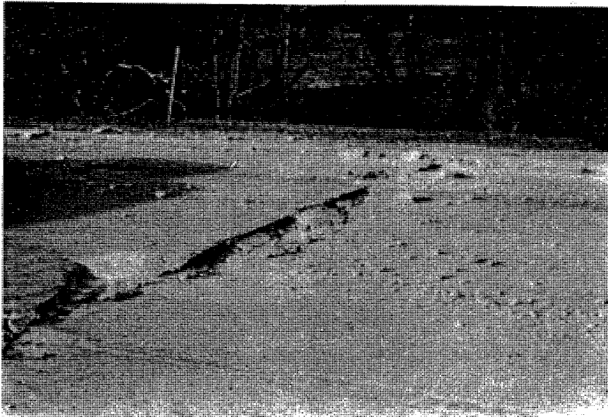
High Severity Shattering Type Blowup
