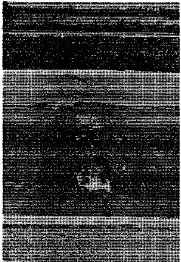
High Severity D-Crack
