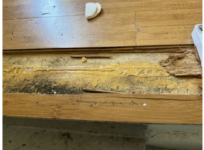
HA-11: Yellow Glue under Wood Laminate Flooring
