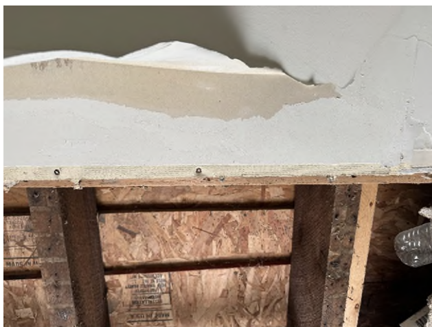
HA-2: White Joint Compound associated with HA-1
