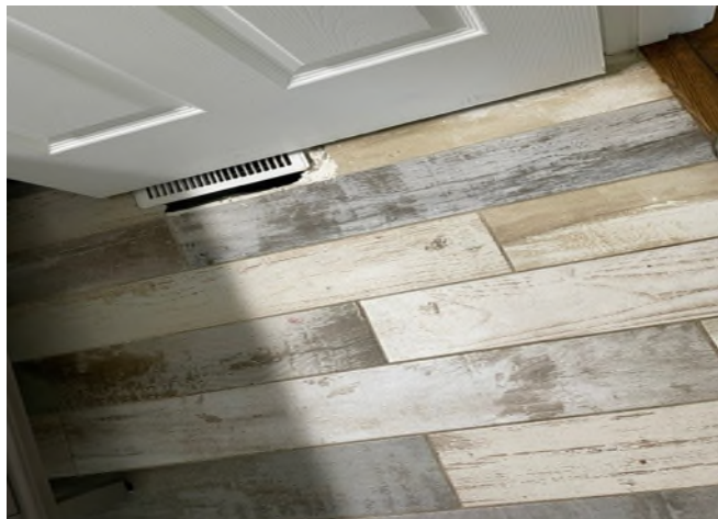
HA-10: White 30" x 6" Wood Pattern Ceramic Floor Tile HA-11: White Adhesive associated with HA-10 HA-12: Gray Grout associated with HA-10
