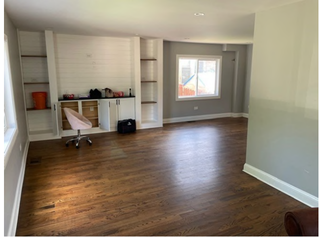
HA-22: Vapor Barrier beneath Hardwood Flooring
