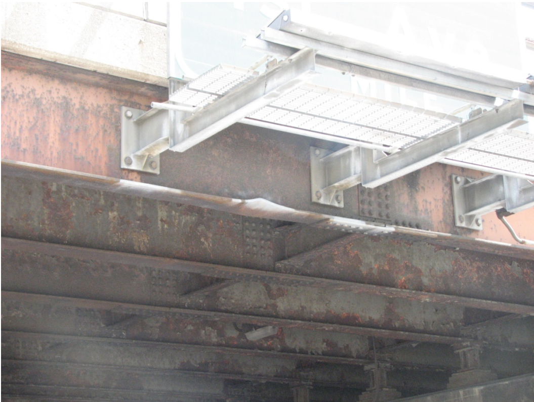
Photo 4 – Signage Supports and Fascia Beam Damage
