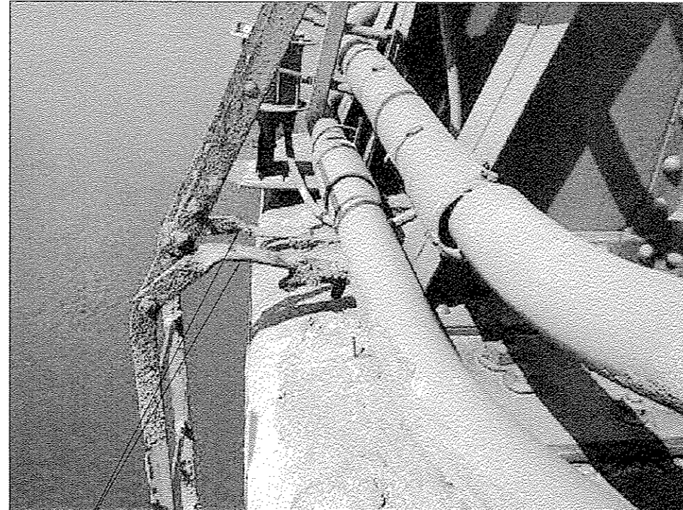
ITEM 612 Ladder at S. end of Pier 9
