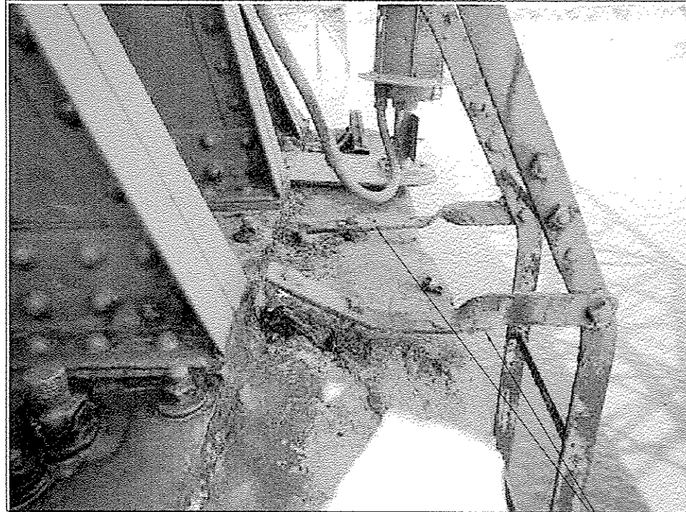
ITEM 611 Ladder at N. end of Pier 9
