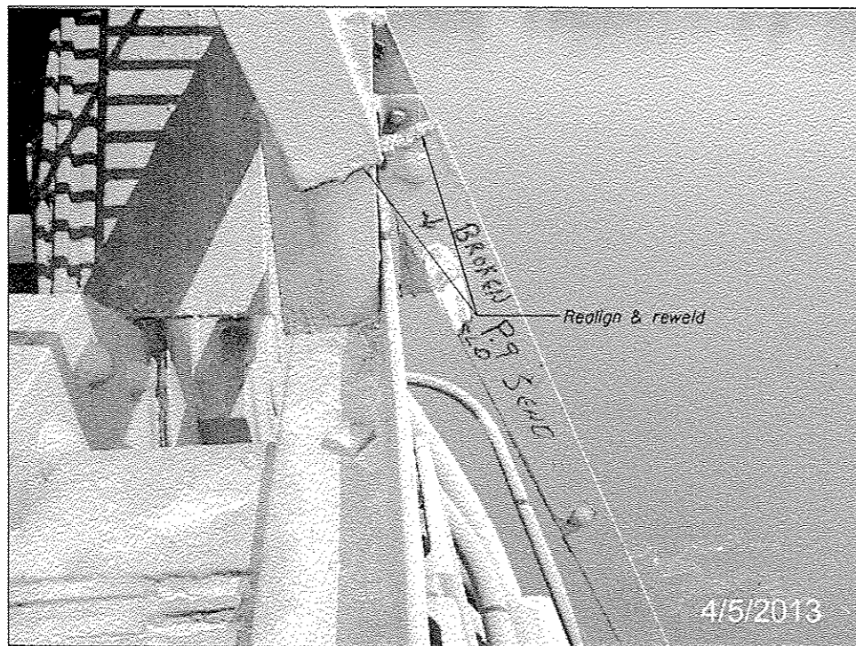
ITEM 612 Ladder at S. end of Pier 9
