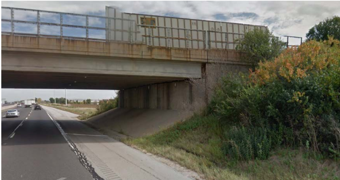
Figure 2: A view to the east-Proposed retaining wall locations on I-55 northbound and Weber Rd abutment
