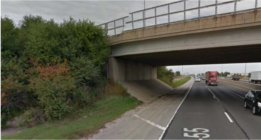
Figure 2: A view to the east-Proposed retaining wall locations on I-55 Southbound and Weber Rd abutment
