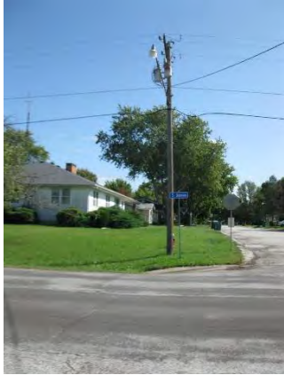
13. Transformer at the corner of Harmony Lane and Johnson Street.
