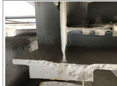
PHOTO #3 SPAN 9 BM GD-3 EF AT PIER D9 NS LKG W (R2)
