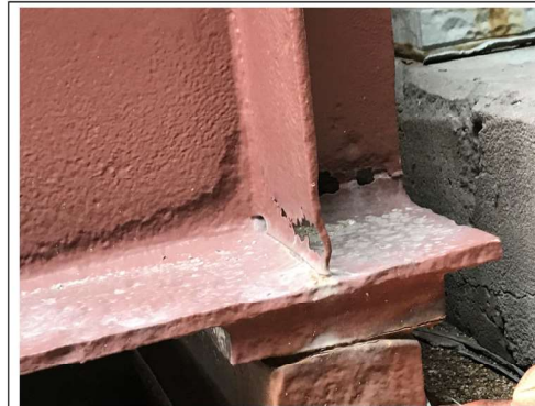
PHOTO #2 SPAN 9 BM GD-2 WF AT PIER D9 NS HOLES LKG SE (R1)
