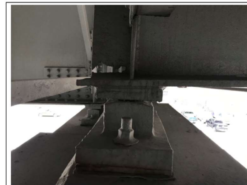
PHOTO #9 SPAN 8 BM GR-11 WF AT PIER D9 SS HOLES LKG E (R5)
