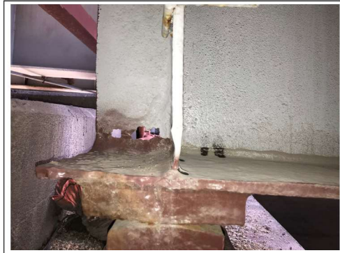
PHOTO #1 SPAN 9 BM GD-2 EF AT PIER D9 NS HOLES LKG W (R1)
