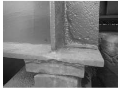
Photo 4: Span 28, Pier 28, G15-L
