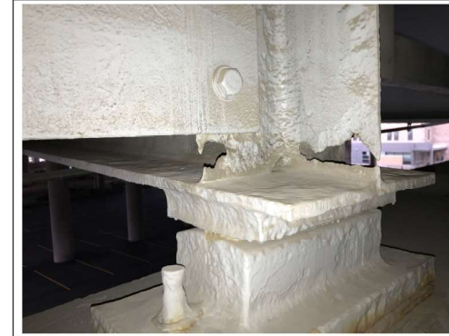
PHOTO #10 SPAN 8 BM GR-11 EF AT PIER D9 SS HOLES LKG SW (R5)
