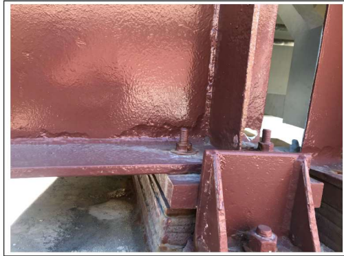
PHOTO #13 SPAN C3 BM GC-1 WF AT PIER C3 NS HOLE LKG SE (R7)
