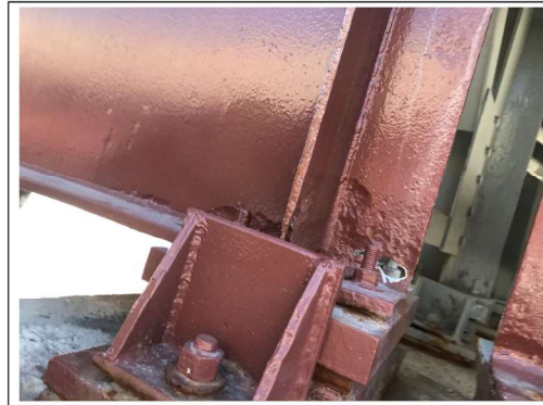
PHOTO #14 SPAN C3 BM GC-1 WF AT PIER C3 NS HOLE LKG NE (R7)
