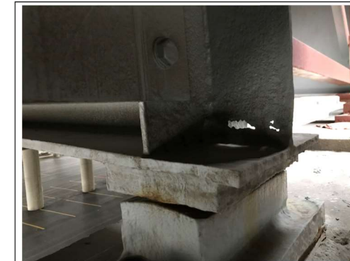
PHOTO #6 SPAN 8 BM GR-10 EF AT PIER D9 SS HOLES LKG SW (R4)
