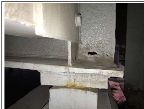
PHOTO #7 SPAN 8 BM GR-10 EF AT PIER D9 SS HOLES LKG W (R4)
