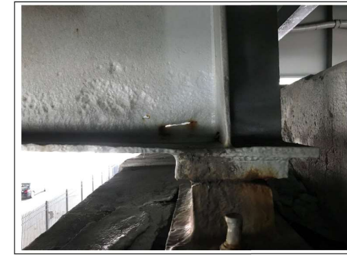
PHOTO #18 SPAN 10 BM GL-1 AT PIER 11 SS LKG W (R10)
