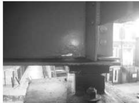
Photo 2: Span 27, Pier 28, G15-L
