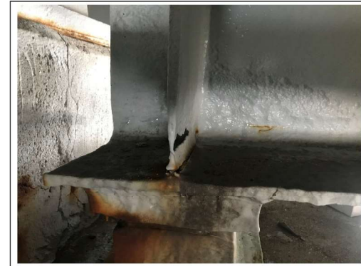
PHOTO #16 SPAN 10 BM GR-1 AT PIER 11 SS LKG E (R9)
