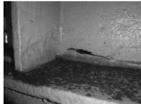
Photo 5: Span 31, Pier 1, G5-L
