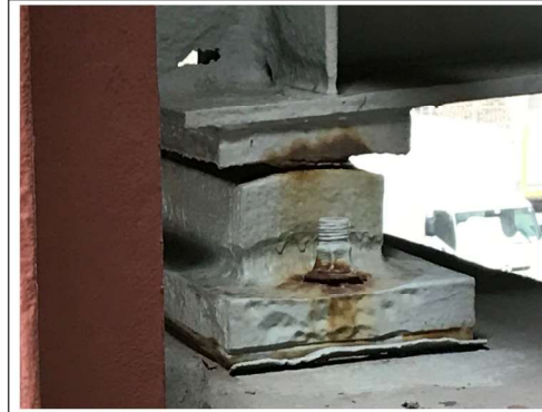
PHOTO #8 SPAN 8 BM GR-10 WF AT PIER D9 SS HOLES LKG SE (R4)
