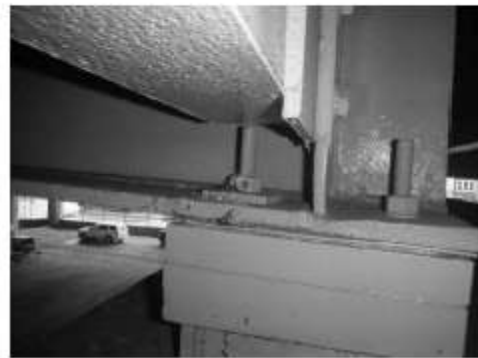
Photo 1: Span 11, Pier 11, G6-L
