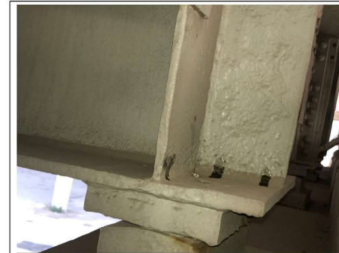
PHOTO #4 SPAN 9 BM GD-3 WF AT PIER D9 NS LKG NE (R2)
