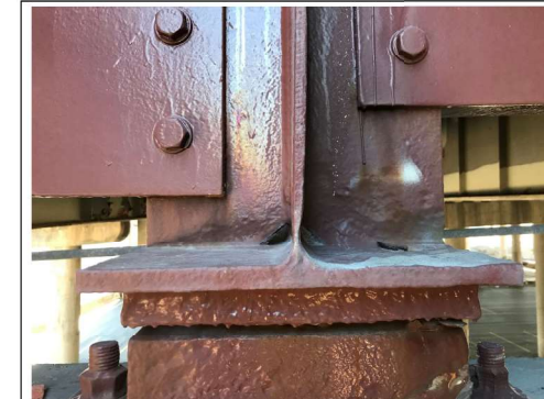
PHOTO #5 SPAN 8 BM GR-9 N END AT PIER D9 SS LKG S (R3)
