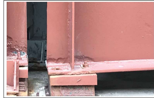
PHOTO #15 SPAN C2 BM GC-1 WF AT PIER C3 SS LKG E (R8)
