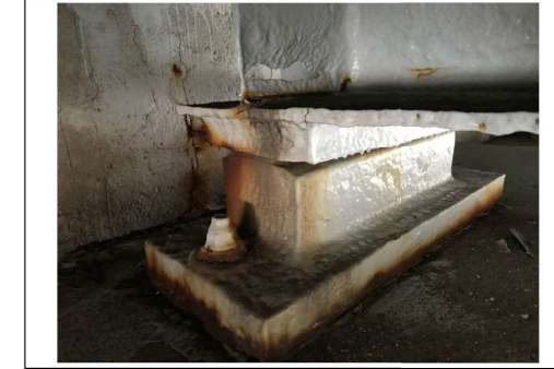
PHOTO #17 SPAN 10 BM GR-1 AT PIER 11 SS LKG NE (R9)
