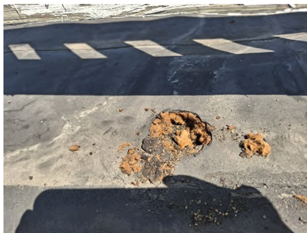
HA-32: Brown Roofing Material under HA-31
