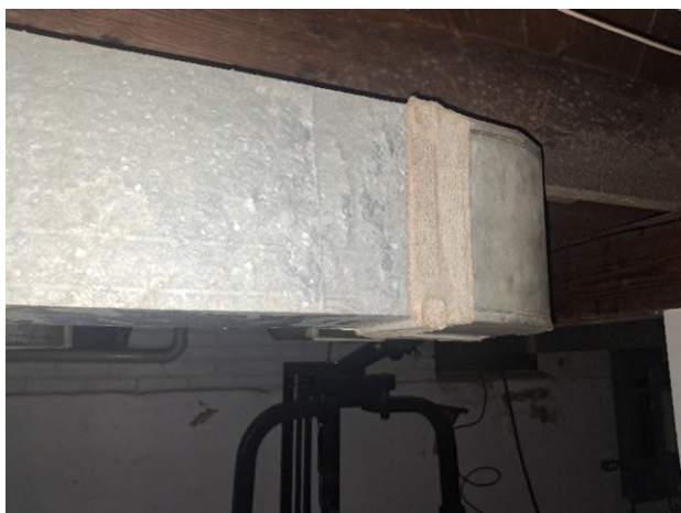
HA-13: White HVAC Duct Tape
