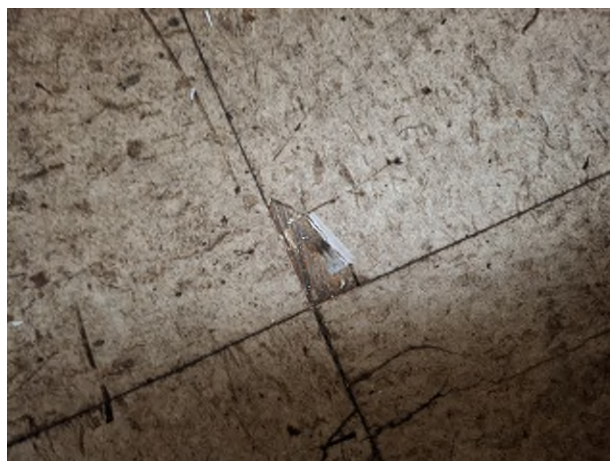
HA-27: Beige 12" x 12" Floor Tile HA-28: Gold Mastic associated with HA-27
