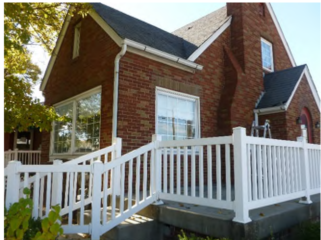
HA-6: White Exterior Window Caulk
