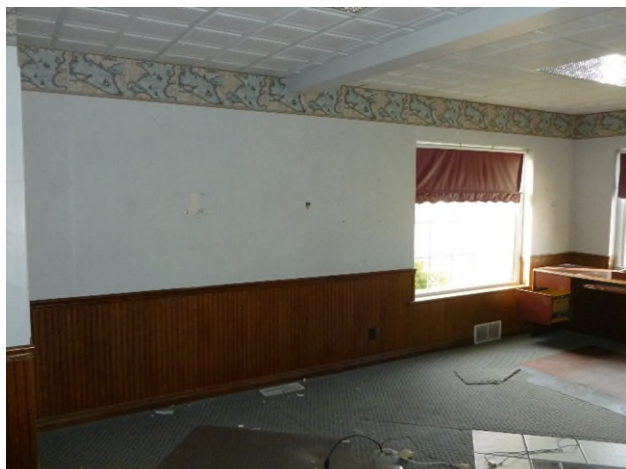
HA-35: White Joint Compound associated with HA-30
