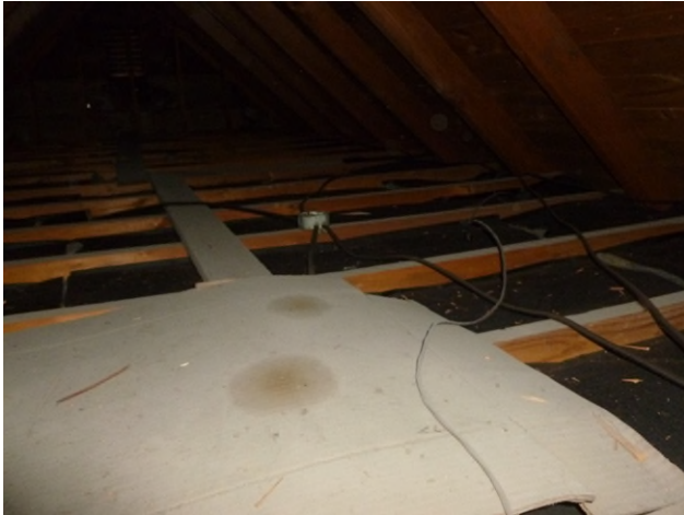
HA-9: Black Cloth Wiring Sheathing
